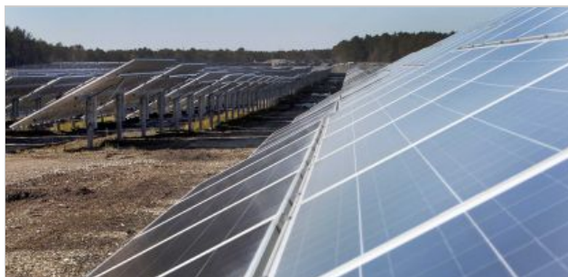
The Long Island Solar Farm in Upton is made up of 164,312 panels that produce 32 megawatts of power. The 200-acre power plant, seen on Nov. 18, 2011, is on the Brookhaven National Laboratory campus. (Credit: Joseph D. Sullivan)
